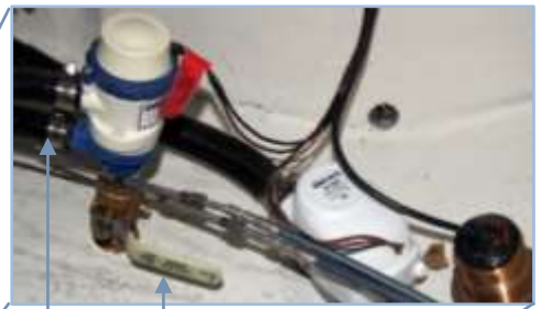
Shut Off Valve
