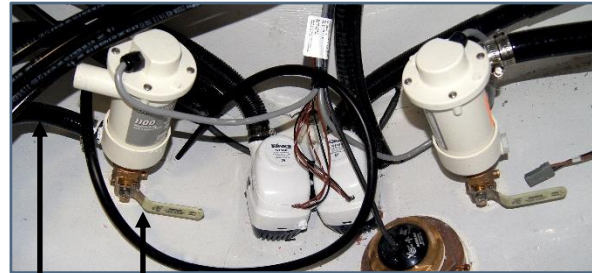
Shut Off Valve
