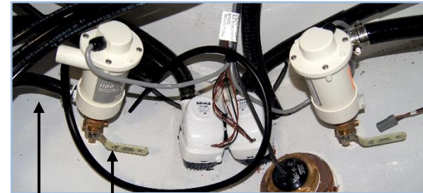
Shut Off Valve
