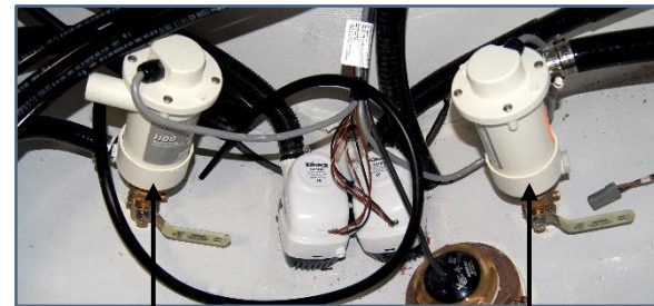
Pumps To Fill Valves
